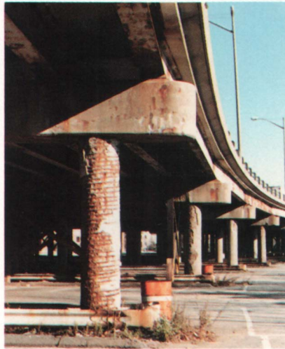
Corrosion of reinforcing steel in concrete (elevated highway, Providence, RI), where road de-icing salts combine with acid precipitation to produce a severe environment. (Photo by Robert Baboian.)
