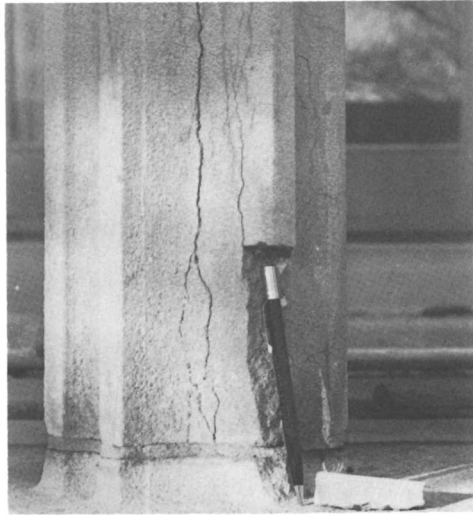
Spalling of marble column on Department of Justice building, Washington, DC. (Photo by Bruce Doe.)
