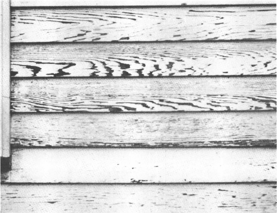
Figure 3.--Paint failure over latewood of flat-grained siding (30). (M147 211-12)
