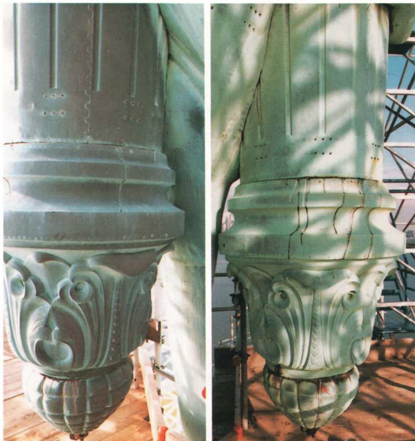
Left side-right side comparison of the Statue of Liberty torch shows darkening of the left side facing Manhattan and the northeast. Darkening of the left side is due to erosion of the green patina by acid deposition and the severe weather from the northeast. (Photo by Robert Baboian.)
