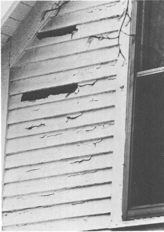
Degradation of paint occurs by reaction at the surface and at the paint interface. Acid deposition can cause paint peeling on wood. (Photo by R. S. Williams.)
