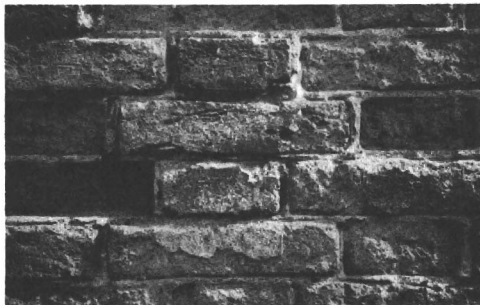
Figure 6. Brick deterioration due to salt crystallization in masonry. In this case the bricks are more porous than the mortar and the salts will accumulate in them leading to their deterioration. Considerable variation in the degree of deterioration is evident.
